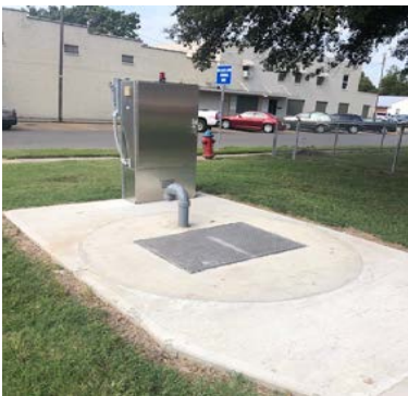
12th & Ward Lift Station
