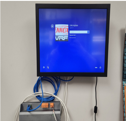
City Hall HVAC
