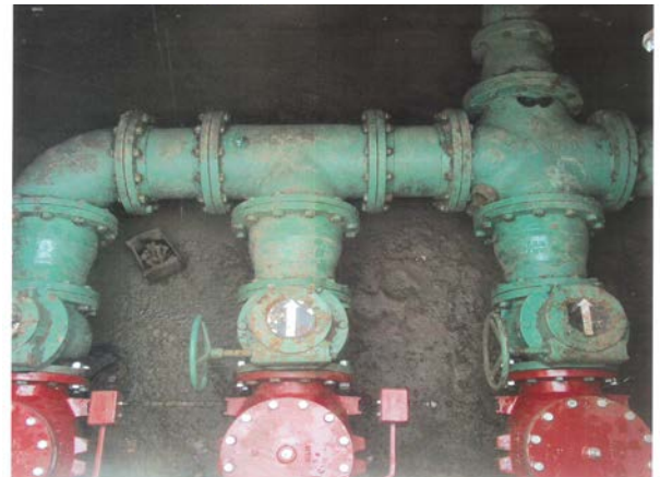
New Check Valves
